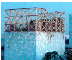
Containment AKW Fukushima
